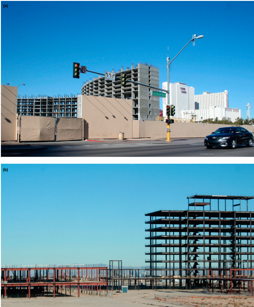
Figure 4. Halted construction projects were unheard of in pre-Great Recession Las Vegas. But, the pause in growth and development were visible in both the tourist core and the suburbs. (a) shows the shell of the first few floors of what was to be Echelon Place, a high-end casino-resort on the Strip's northern end. (b) is the abandoned frame of a suburban shopping mall at the Las Vegas Valley's western edge. Photos by author, January 2011.
